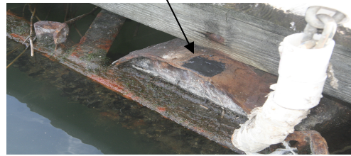
Rust hole in float
